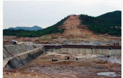
Construction work takes place Friday, June 28, 2013, at the site of the planned Grand Ethiopian Renaissance Dam near Assosa in the Benishangul-Gumuz region of Ethiopia, near Sudan, some 800 kilometers (500 miles) from the capital Addis Ababa. (AP Photo/Elias Asmare)
