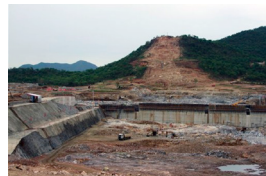
Construction work takes place Friday, June 28, 2013, at the site of the planned Grand Ethiopian Renaissance Dam near Assosa in the Benishangul-Gumuz region of Ethiopia, near Sudan, some 800 kilometers (500 miles) from the capital Addis Ababa. (AP Photo/Elias Asmare)
