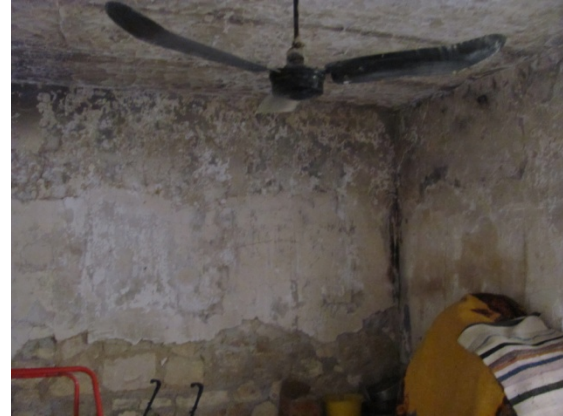
Figure B-4. Burned interior of Jassim's brother's house next door
