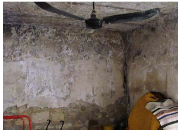
Figure 2-8. Burned interior of Jassim’s brother’s house 41
